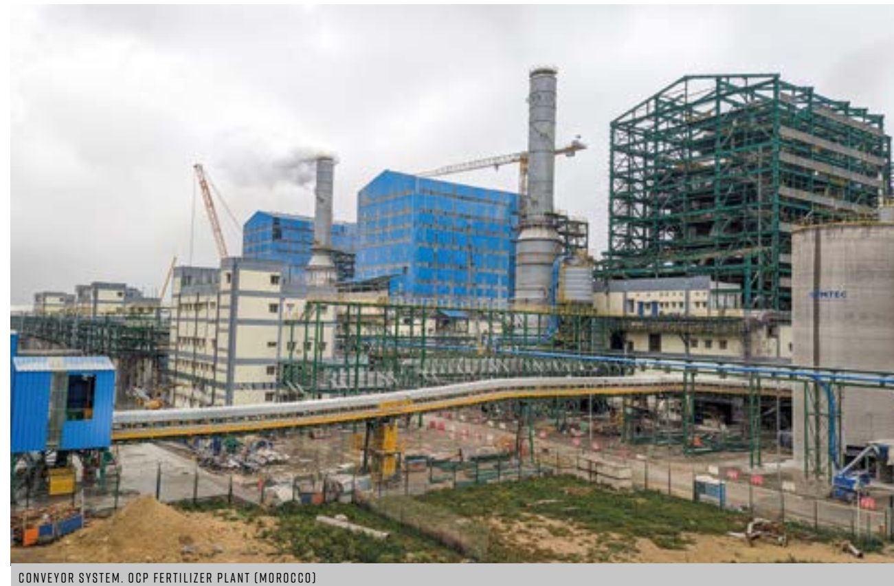
CONVEYOR SYSTEM. OCP FERTILIZER PLANT (MOROCCO)
