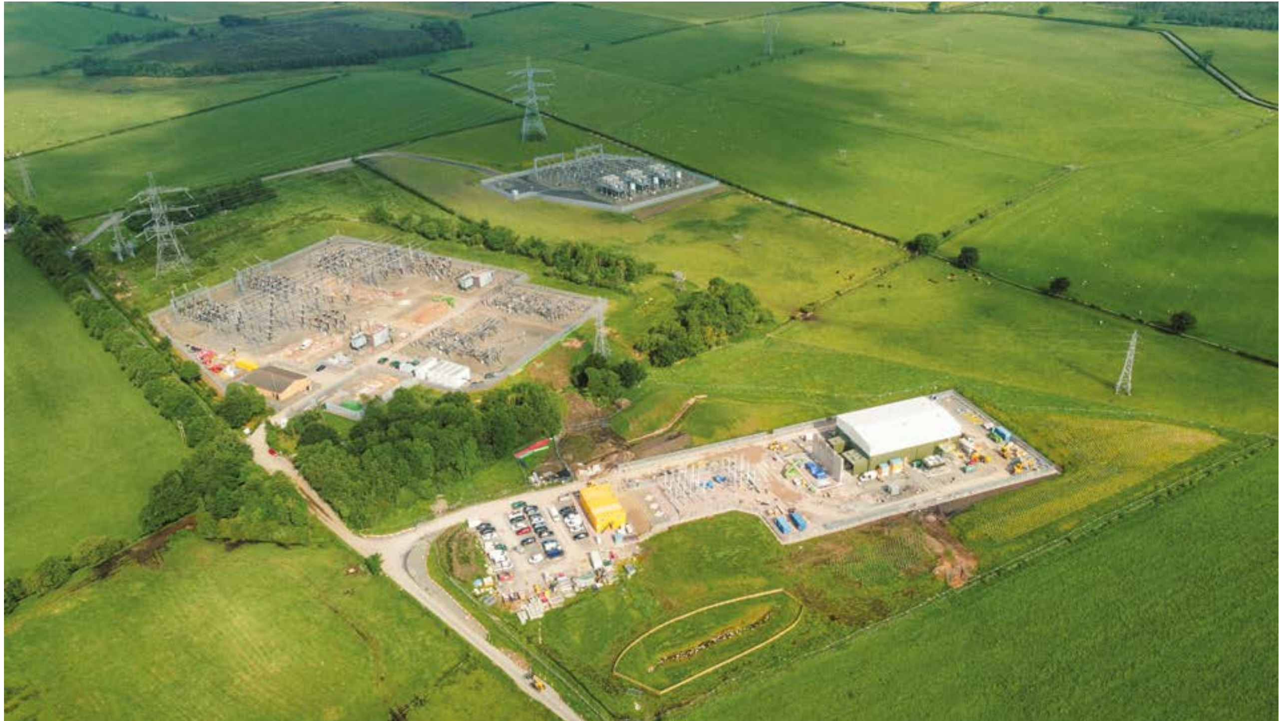
GRID STABILITY PLANT GREтна (UNITED KINGDOM)
