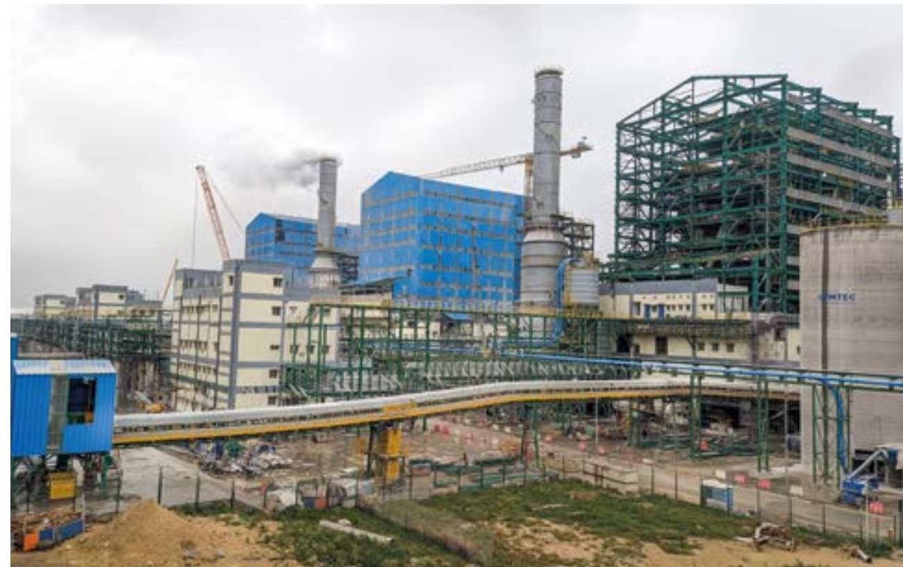
CONVEYOR SYSTEM. OCP FERTILIZER PLANT (MOROCCO)
